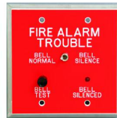
Fire Alarm Trouble
