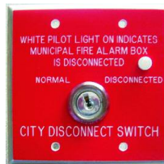
City Disconnect Switch
